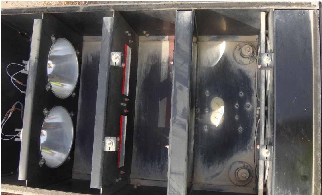
A similar unit that has been cleaned, with no loose dirt, just about to an acceptable standard. Note the reflectors showing signs of deterioration- scratching and oxidation.
