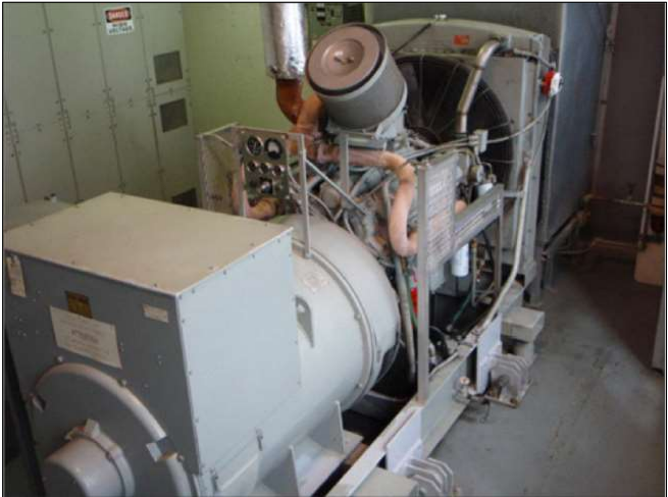
Figure 2-7. Diesel-electric generator set (source: Toronto International Airport)
