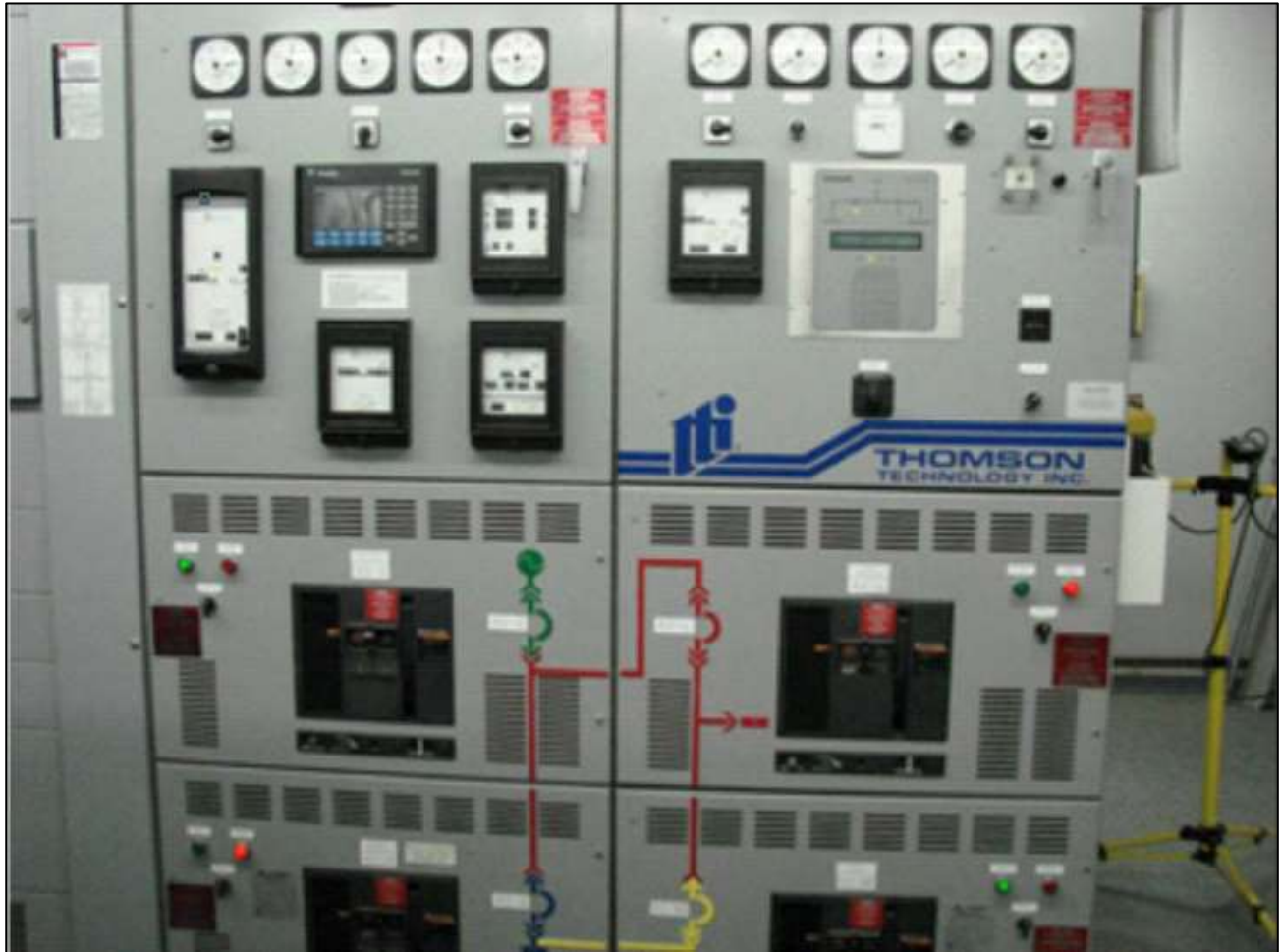
Figure 2-8. Transfer panel (source: Toronto International Airport)
